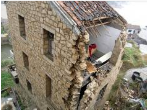
Fig.9 Collapsed stone house
