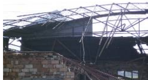
Fig.14 Damage to work shed
