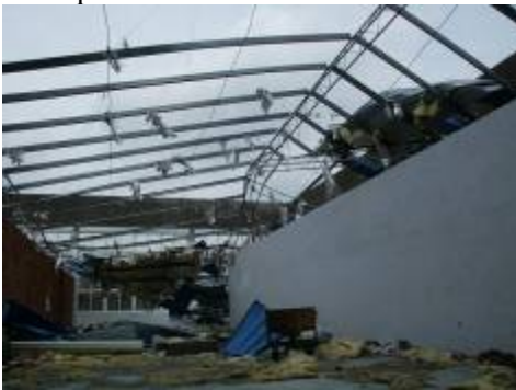
Fig.11 Damage to factory building roof
