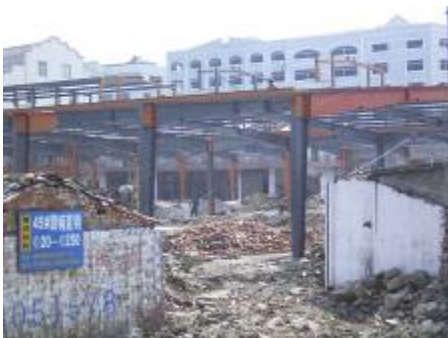
Fig.13 Roof completely destroyed
