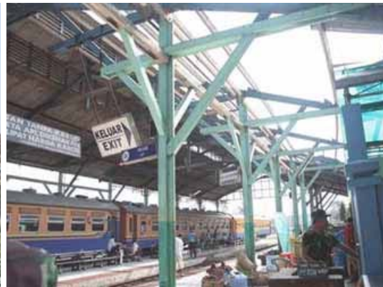
Figure 6. Damage to Station Hall
