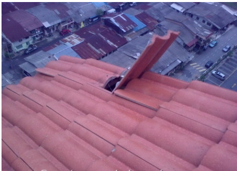
Figure 4a: Uplift Roof Tile
