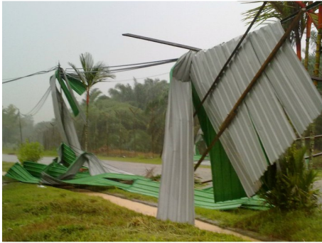
Figure 1c – Roof Sheet Failure
