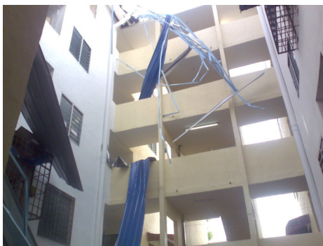
Figure 1a – Steel Truss failure
