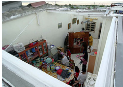
Figure 1d – Roof Damage
