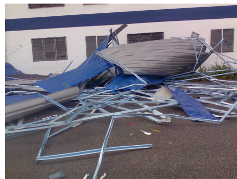
Figure 1b – Steel Truss failure
