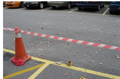
Figure 4d: Flying Debris of Roof Tile
