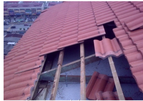
Figure 4b: Damage Roof Tile
